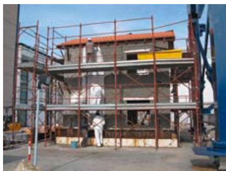
Experiment in Pavia: A badly damaged building is reinforced with the seismic carpet to be placed on a vibrating table for testing the intelligent composite seismic wallpaper.
